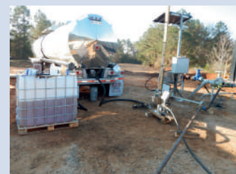
Formulation truck directly connected to injection pump for in-line mixing and direct injection of the foaming formulation.
